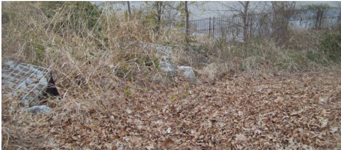
PROBLEM Gabion baskets were failing to provide stability at the Metal Art Museum
