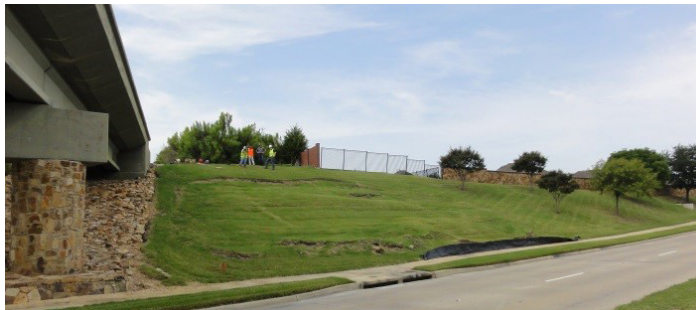
PROBLEM Roadway and railroad bridge embankment slope failure
